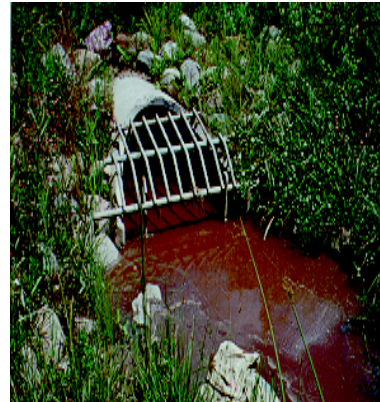
Typical Inlet Pipe
