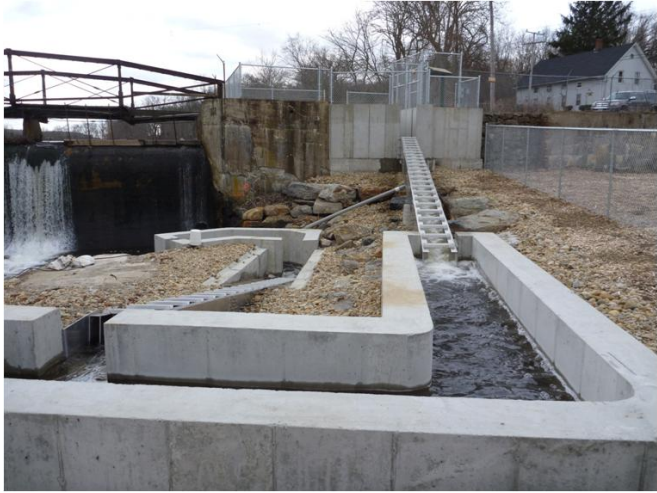
The Shewville Dam steppass fishway will be the same type of fishway installed down river at Hallville Pond.
