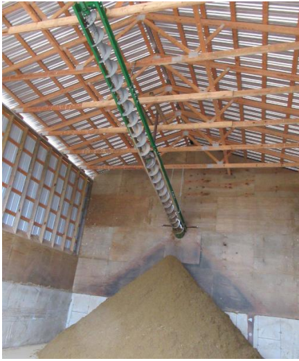
A screw auger moves bedding from the liquid-solid separator to the storage room.
